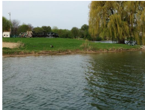
An eroding shoreline at Candlewick Lake (left).
